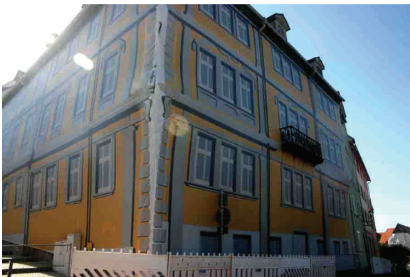
Look closely – this is actually a tarp, maintaining a nice, cohesive look during renovation
