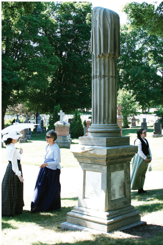
Project complete! The Dickinson Monument cleaned and with the top section back in place.
